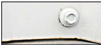
Environmental tests show extensive corrosion along cut end of panel without Edge-Rust Inhibitor.
